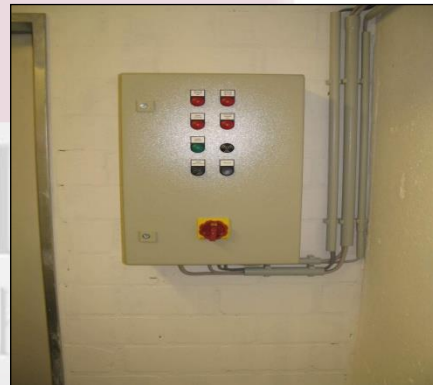
Control cabinet for MA-3000
