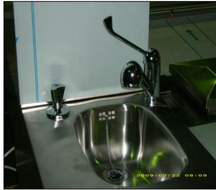
Sink with 25mm radius, elbow operated taps with flexible hose 1500mm long. Left: Valve for operation of sprinkler system below work area
