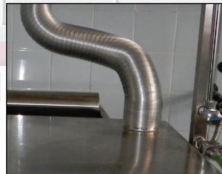
Connection to inhouse ventilators
