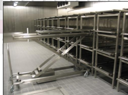
MA-1307 Support racks for large volume storage at a cold room Note fridge unit at the upper wall / ceiling
