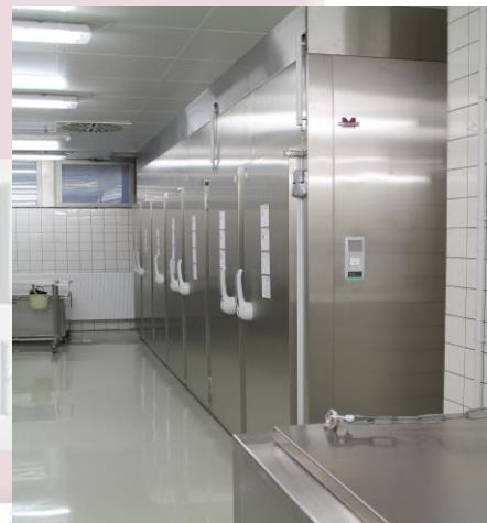
MA-1239 Deep freeze rooms, 4-tier (-20°C)
