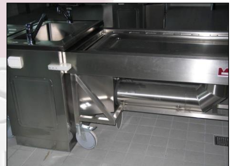
Air extraction duct
